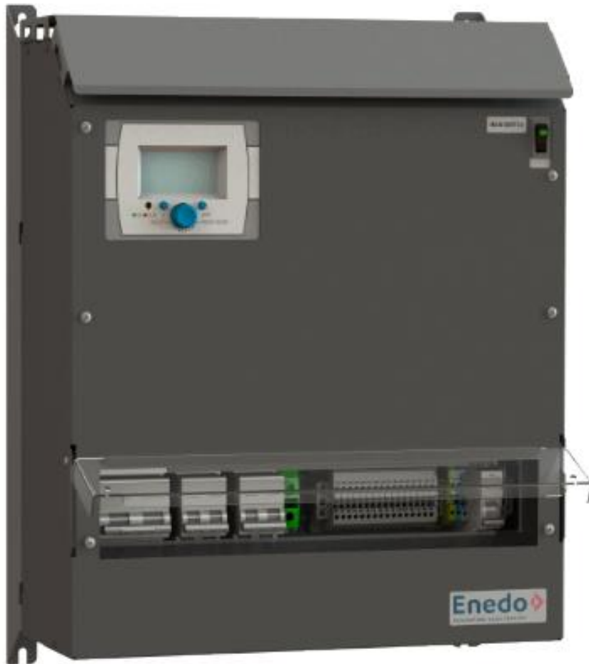
Figure 5. Normal operating mode, system cover installed, operational switches and local UIF display available
