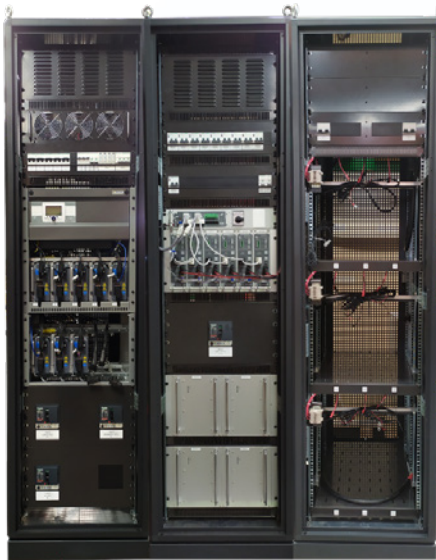
16kW Multi-Output DC Power System with Battery Backup for an Oil & Gas production facility requiring different voltage levels
