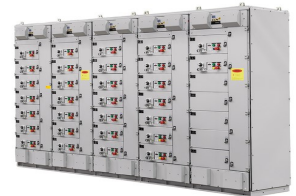
Motor control centres LV
