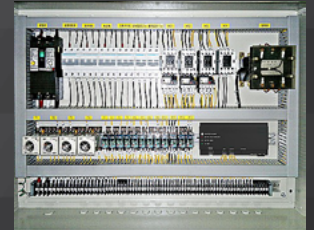
Power control cabinet
