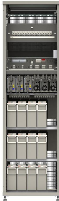
OPUS HE 48-6.0 OC2066 48VDC 41.7A – 125A DC/DC Converter up to 3 x 750W 2 x MCB 125A battery fuses Battery & distribution space
