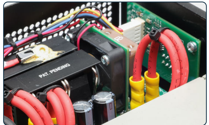
Cooling fan location.
