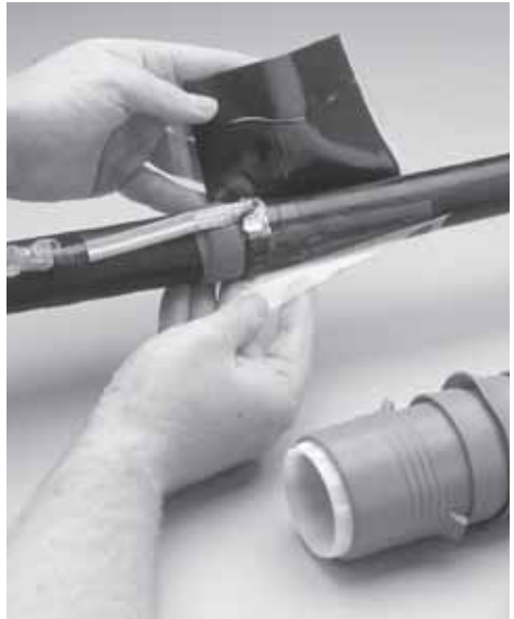
Photo 7: Applying the stress control patch. In line with initial outer layer cut and over the bonding braid.
